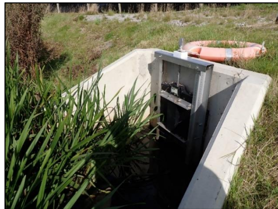
This is the closure device on the outlet from the pond. This can be closed in the event of a spill or an accident.
